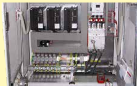
Switchgear with thyristors in phase angle operation for economic power consumption
