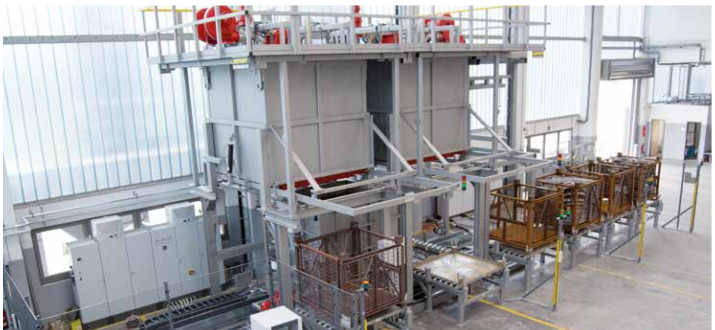
Fully automatic drop-bottom furnace plant, consisting of two drop-bottom furnaces, movable water bath and several loading and unloading positions
