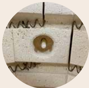
Thermocouple positioned in insulation as protection
